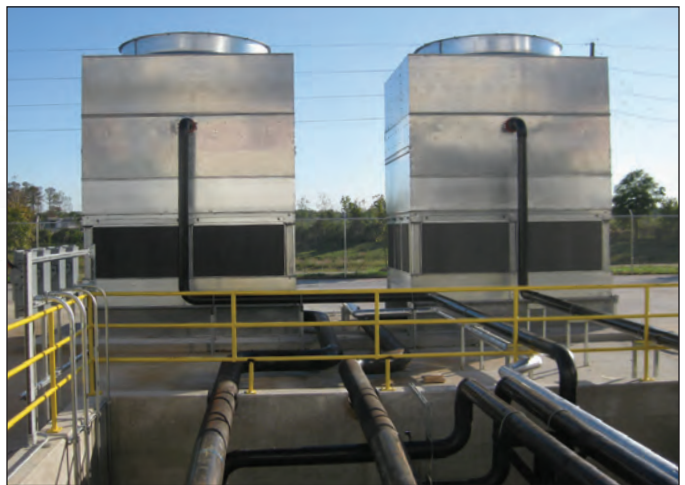
Cooling Towers for below grade system
