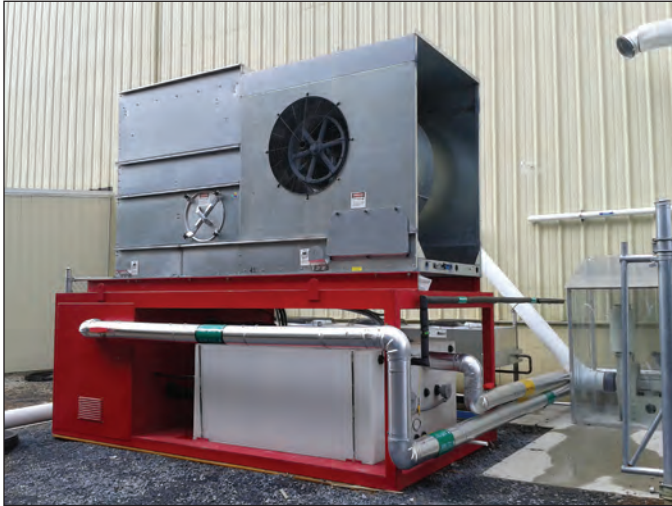
Above ground packaged WRS
