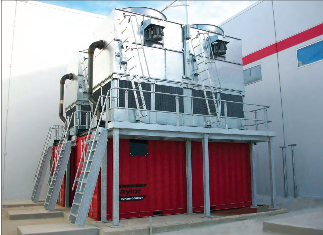
Above ground Containerized Water Recirculation System
