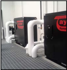
Coolant Storage and Distribution
