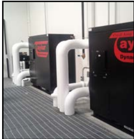
Coolant Storage and Distribution
