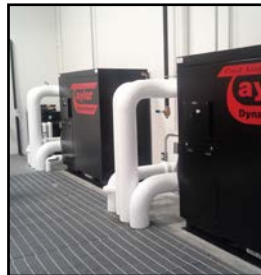
Coolant Storage and Distribution
