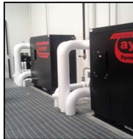
Coolant Storage and Distribution
