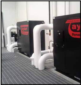
Coolant Storage and Distribution
