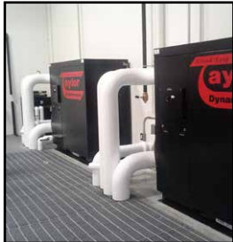
Coolant Storage and Distribution
