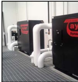
Coolant Storage and Distribution
