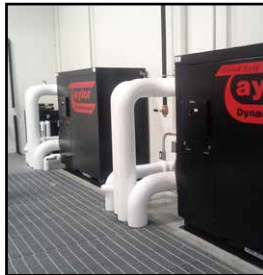
Coolant Storage and Distribution
