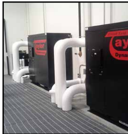
Coolant Storage and Distribution
