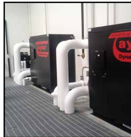
Coolant Storage and Distribution
