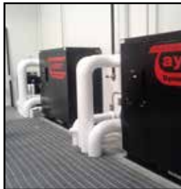
Coolant Storage and Distribution
