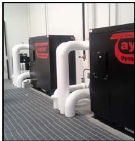
Coolant Storage and Distribution
