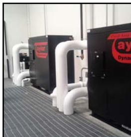
Coolant Storage and Distribution
