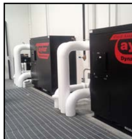
Coolant Storage and Distribution
