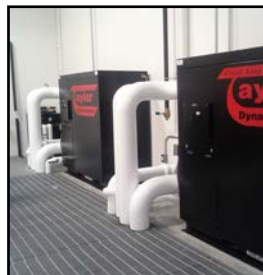
Coolant Storage and Distribution
