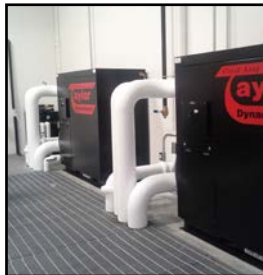
Coolant Storage and Distribution
