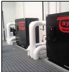
Coolant Storage and Distribution
